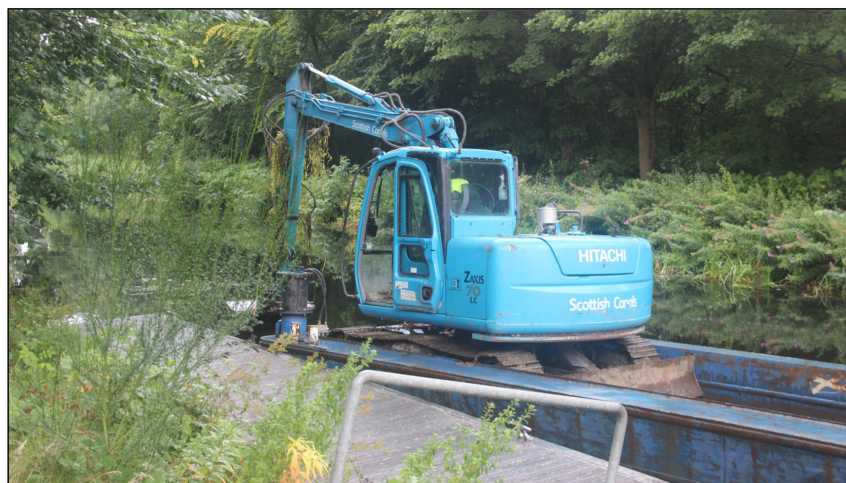
Figure 4. Barge-mounted excavator in operation on the Forth & Clyde Canal at Old Kilpatrick, September 2020.
