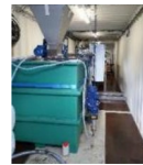
Flocculant preparation zone
