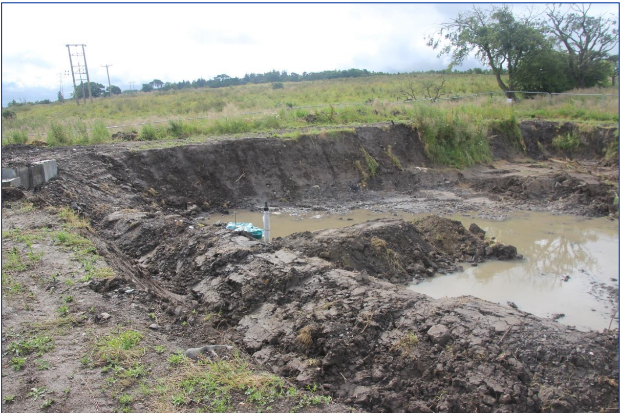
Figure 18. Construction of earthen bund along the northern side of the treatment cells.
