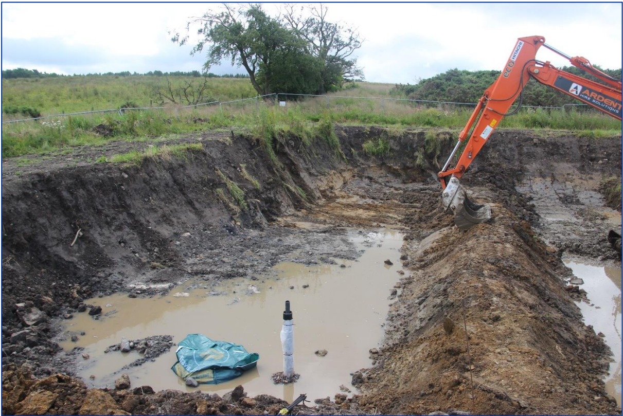
Figure 19. Cell F1 after construction of the bund separating it from cell F2.
